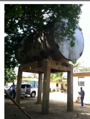
Figure 4: Batey 22 source tank serving Batey 22 and Batey Tentación
